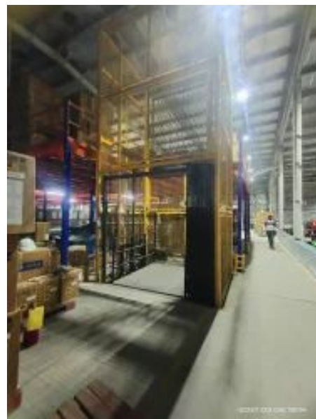
Hydraulic Goods Elevator
