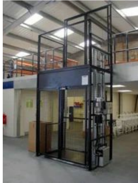
MS Goods Elevator
